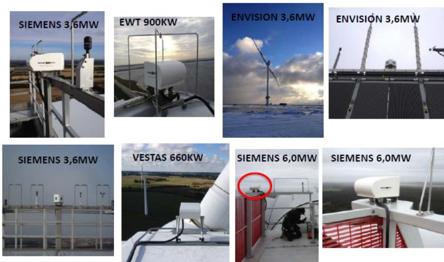
Fig. 9. Images showing some of the current turbine installations of WindEye sensors.
