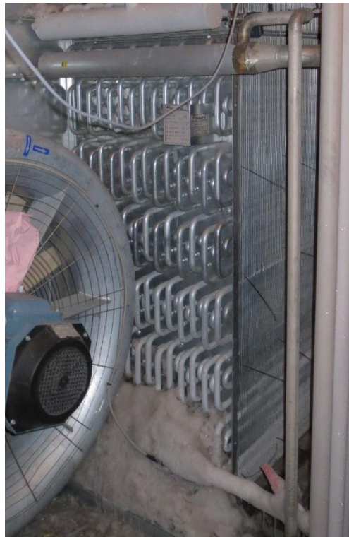
Figur 5-8: Fordamper 1 i tunnel 2
