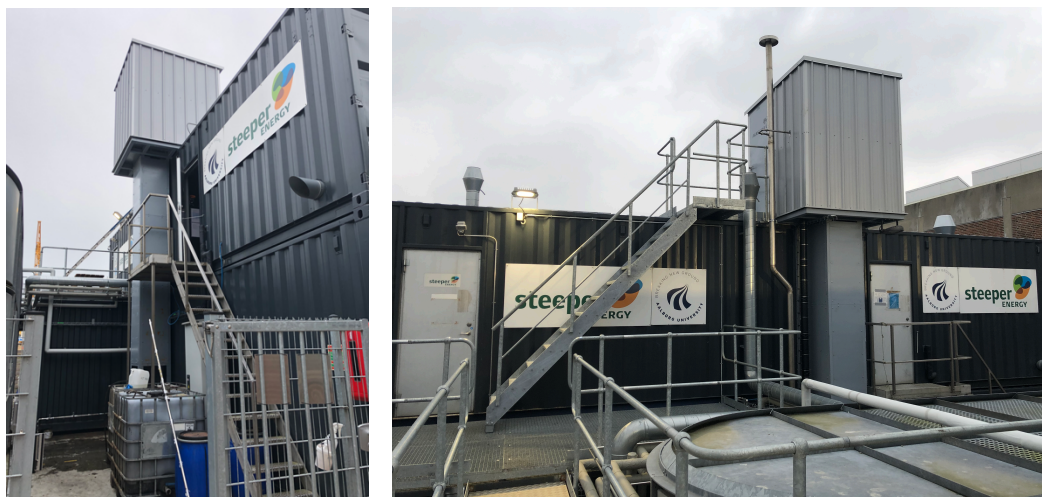
Figure 13: New reactor installation at the pilot plant at Aalborg University.
