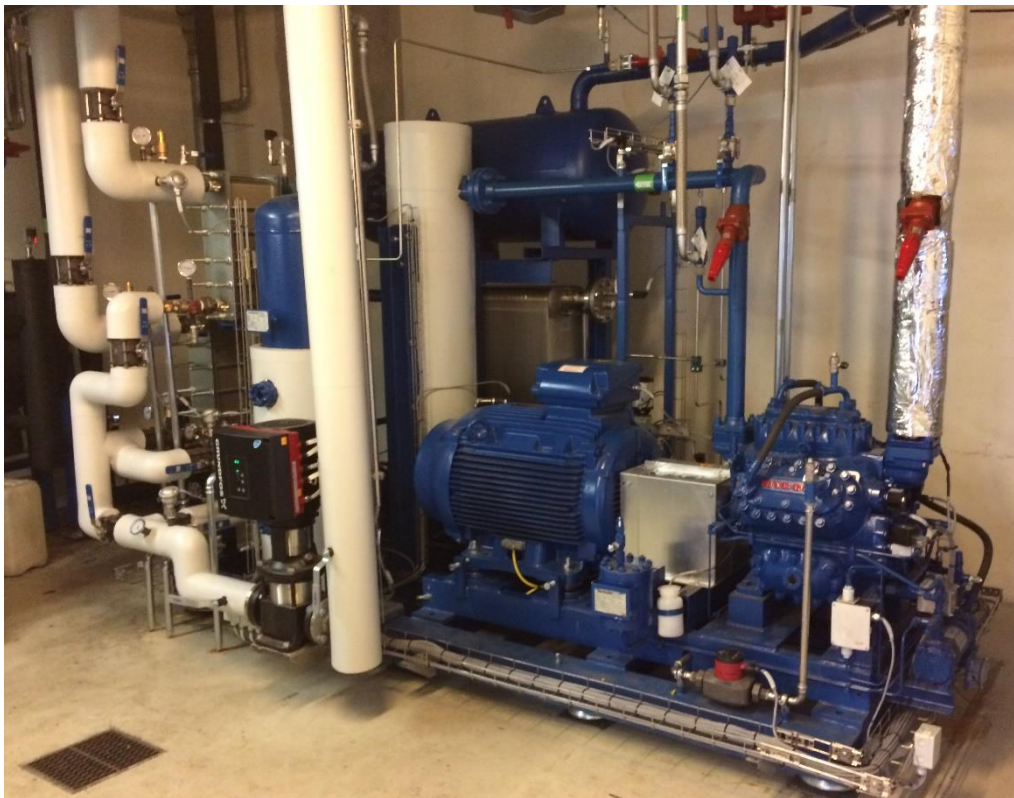
Figure 35. Heat pump installation in Frederikssund, Denmark, with split condenser.
