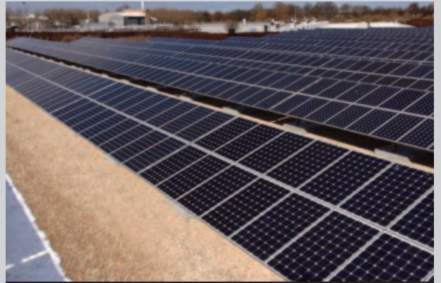
777 kWp PV at Damhusåen waste water treatment plant. Photo by Jon Rytter
