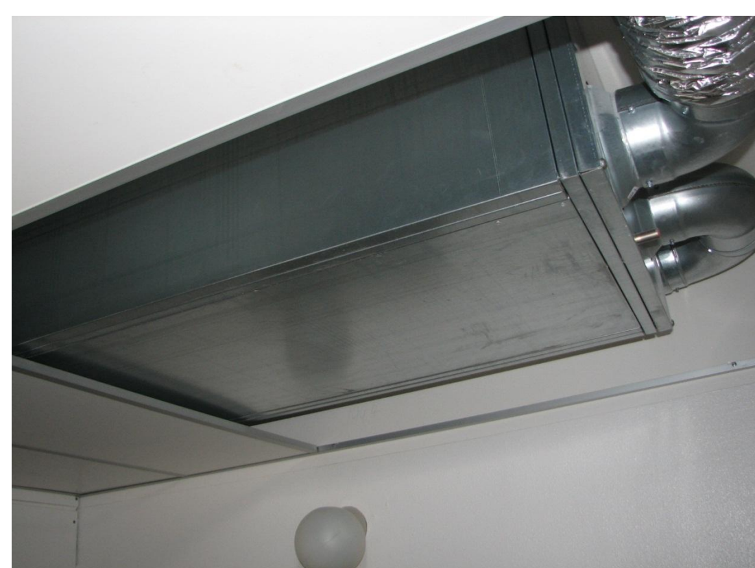
PV-ventilation. Compact Heat Recovery Ventilation for housing renovation where electricity use is matched by BIPV
