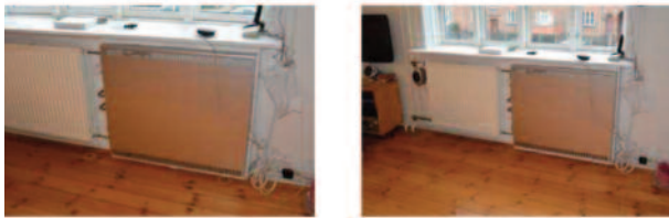
A very well-functioning example of window integrated heat recovery ventilation (HRV) was established at the P. Knudsens Gade housing area, administered by the housing association AKB, in Sydhavnen in Denmark situated in the Concerto area of the Green Solar Cities EU-Concerto project in Denmark.
