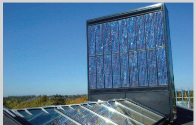
Solar chimney, Lundebjerg, Skovlunde was result of architectural competition with focus on PV and ventilation.
